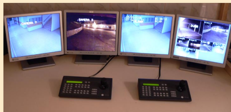
▲ Total overview on the monitors
